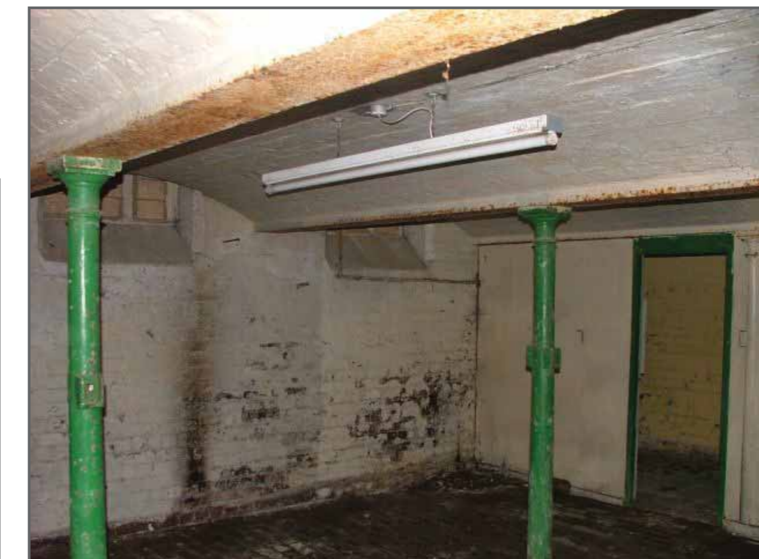
Left: The roof of the basement (located underneath the Church of England chapel) comprises four bays of brickwork vaulting supported by iron joists and cast iron columns.
