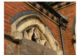
Defective hood mould and tracery
